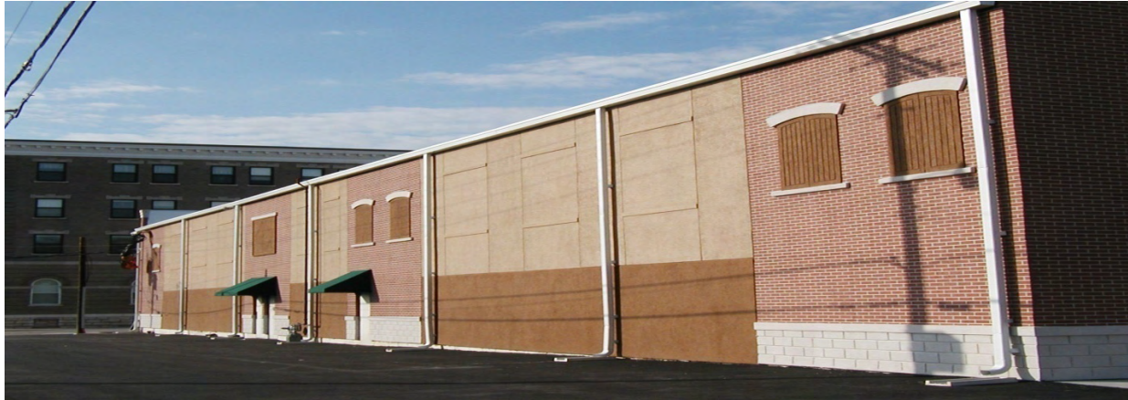
The Dryvit Outsulation System used on the rear of the building shows "fake" boarded up windows, sills and docks along with a variety of surface treatments.
